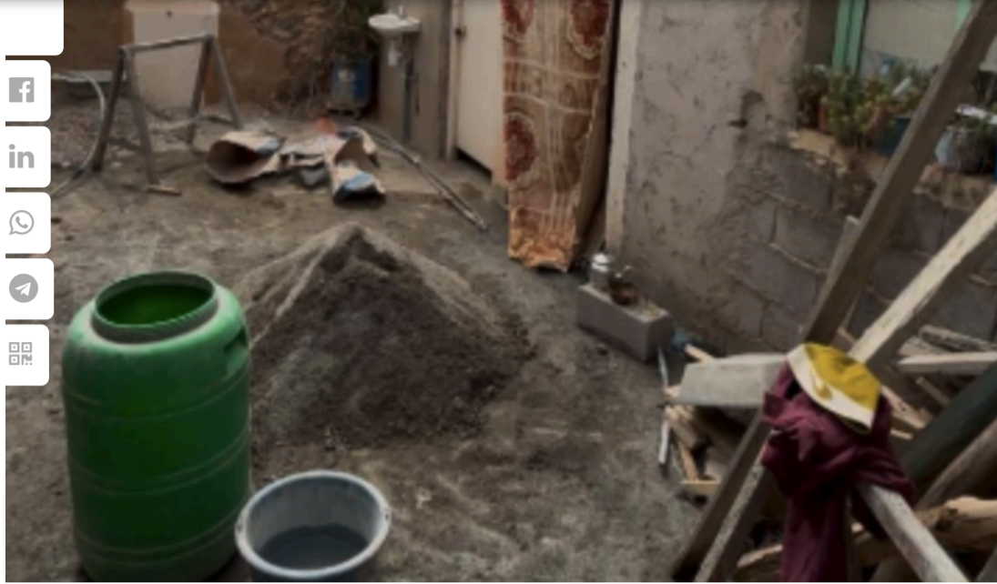
Incomplete post-earthquake reconstruction in Amizmiz. (Credit: HUD student Project, 2025)
