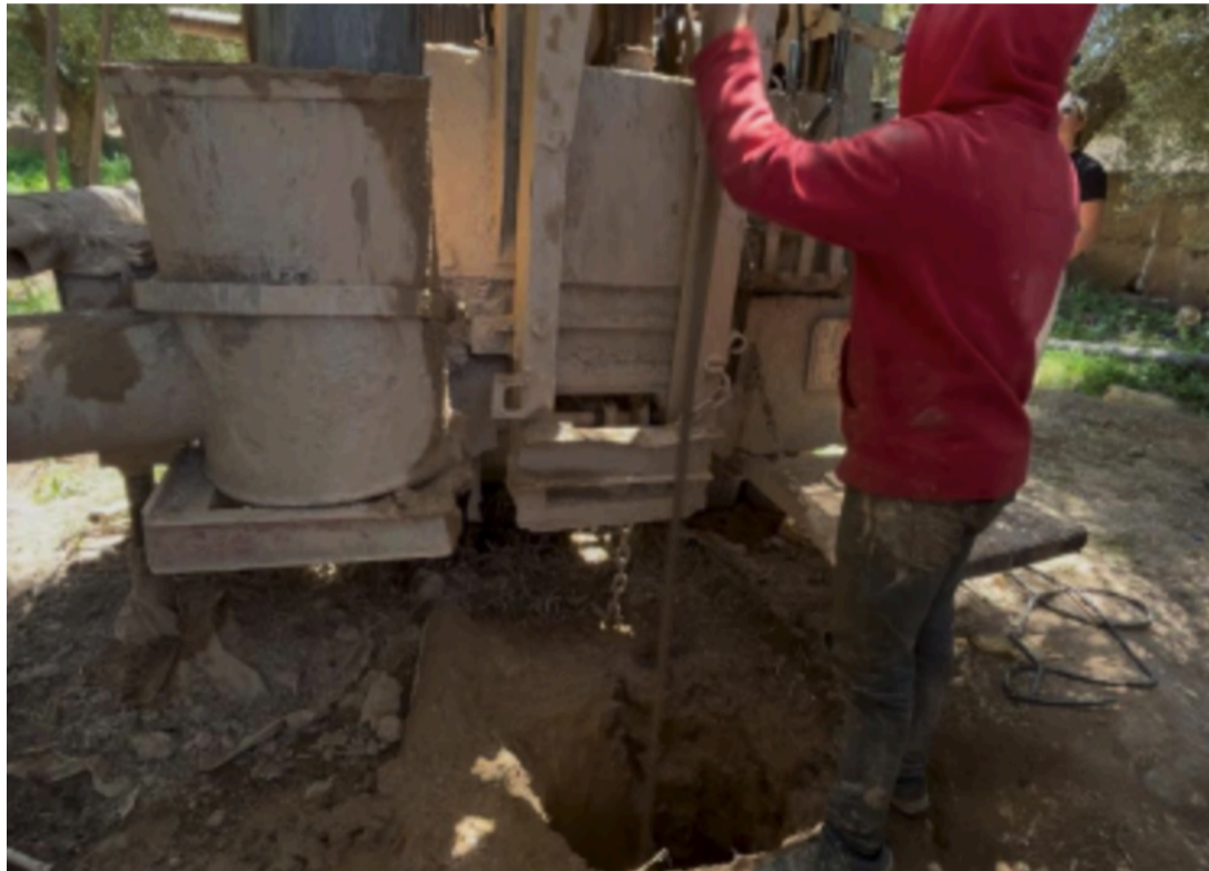
A local worker drills a well in Amizmiz. (Credit: HUD student Project 3, 2025)
