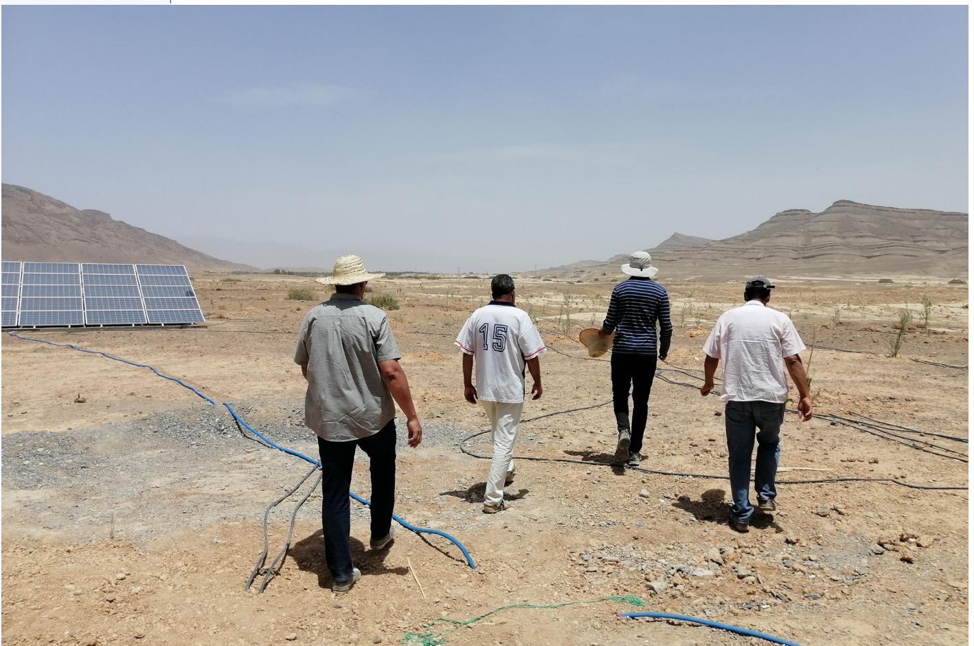
IMAGE 1 | Solar-powered drip irrigation is a zero-emission technology that provides water efficiently for agricultural use.
