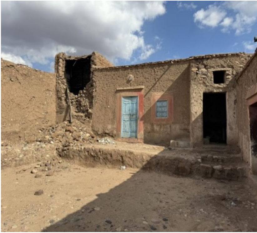
Figure 19 Partially damaged house.
